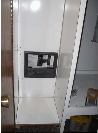
Electrical Panel Mounted
